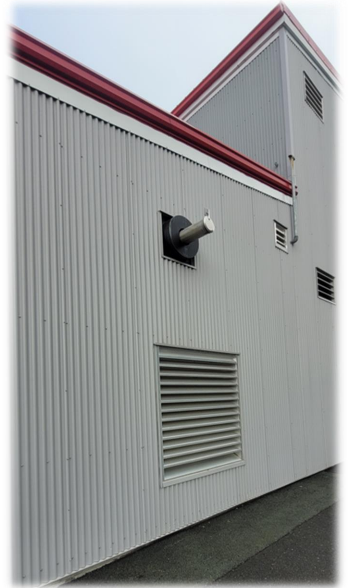
MSH backup generator exhaust and vents
